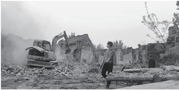
Figure 6. Li Yang. Ancestral House Being Demolished . Video clip. South Slope Yangjia Village, Jiuhu Town, Zouping City, Shandong Province, China, April 18, 2020.
