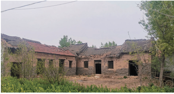
Figure 5. Li Yang. Ancestral House (built in the late 19 th century). Photograph. South Slope Yangjia Village (坡南楊家村), Jiuhu Town, Zouping City, Shandong Province, China, April 18, 2020.
